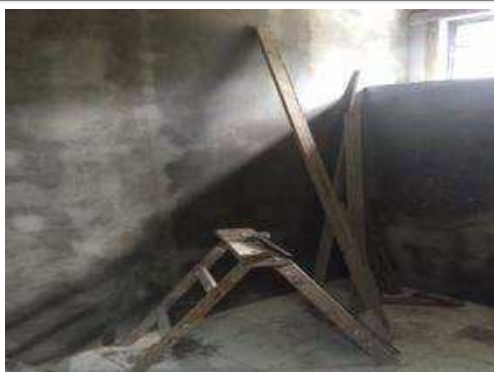
Reboco antigo bwc PNE
